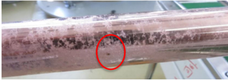
FIG. 18. Inlet cooling pipe of the second coupler of C-ADS Injector I RFQ leaked possibly resulting from strong multipacting.
