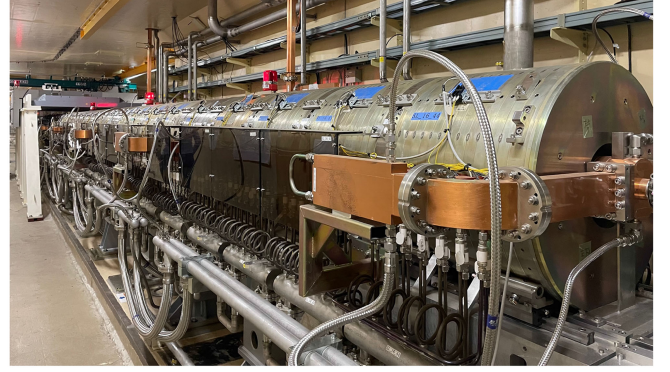
FIG. 10. SuperKEKB e^+ capture section. Photographed in November 2023 during the maintenance day.
